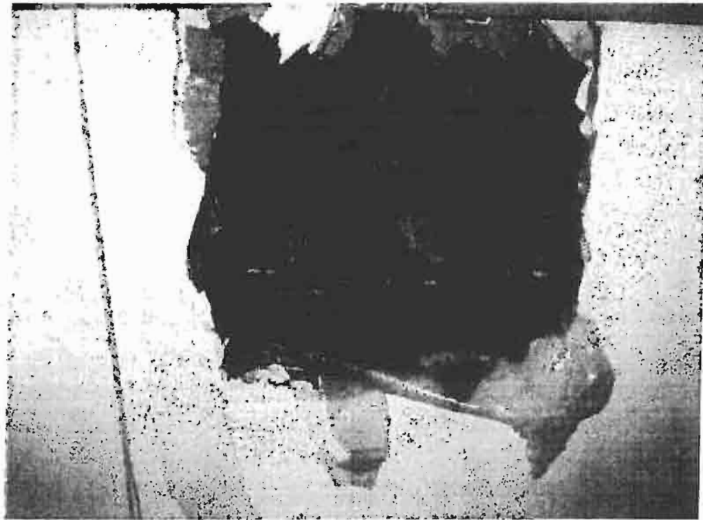
Photo No. 15: Hole through Interior Finishes showing Original Wall Finish and Brick Wall. (2014-05-23)
