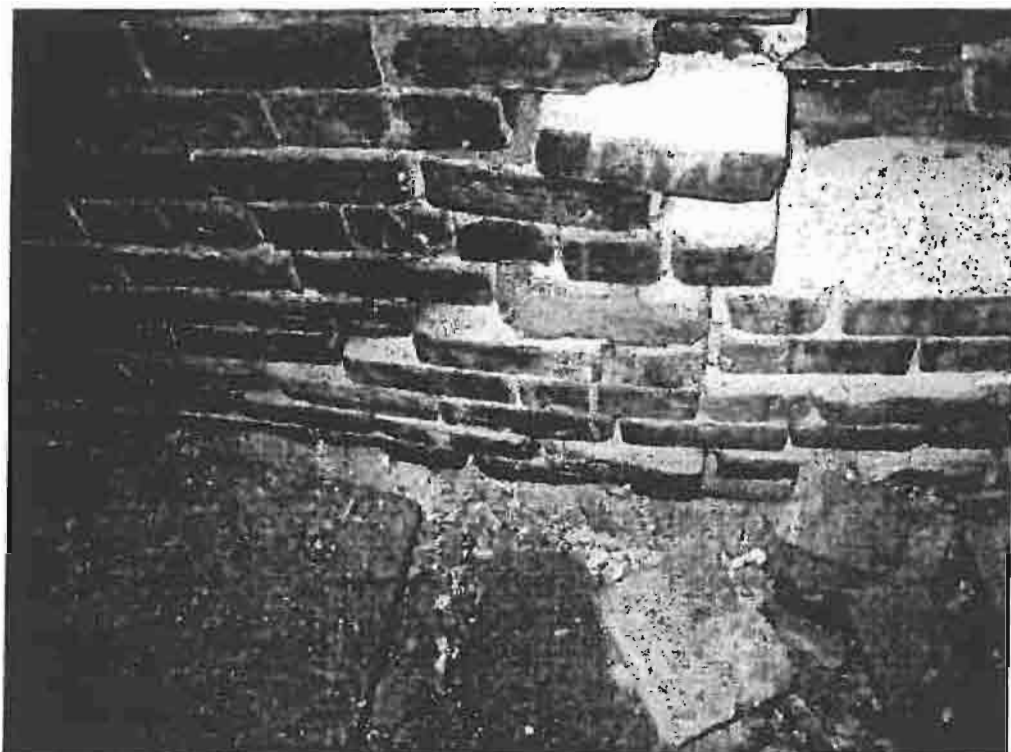
Photo No. 12: Upper East Wall. Brick Failure inside Attic Space. (2014-05-23)
