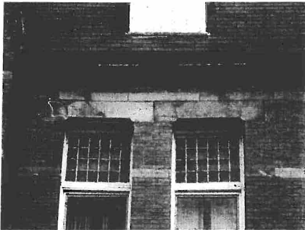
Photo No. 5: Back of Building – Movement of Lintel over Windows. (2014-05-23)
