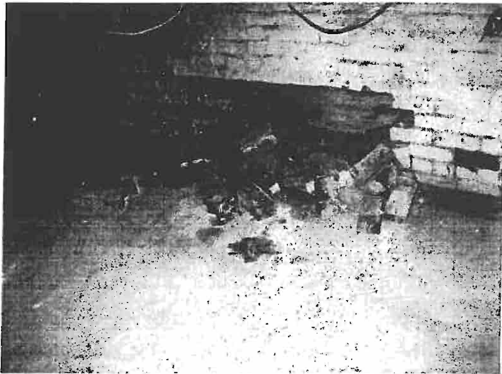
Photo No. 14: Failure of Lower Load-Bearing Brick Wall in Basement. (2014-05-23)
