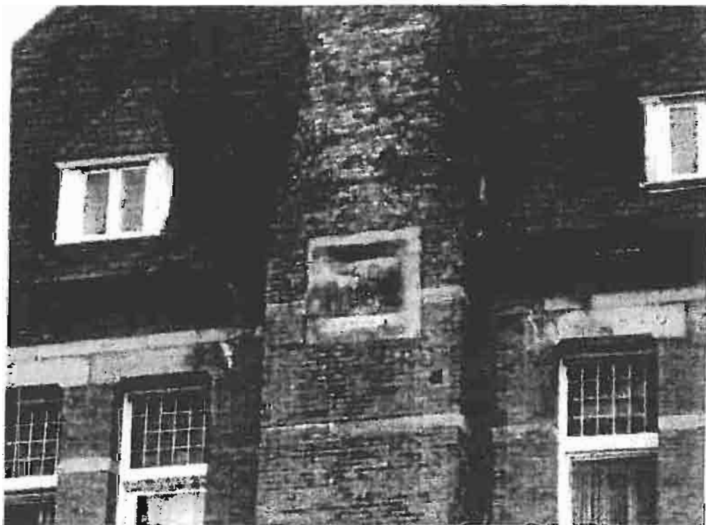
Photo No. 4: Back of Building – Brick Deterioration. (2014-05-23)
