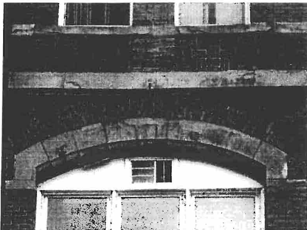
Photo No. 6: Back of Building – Movement and Deterioration of Lintels and Brick. (2014-05-23)
