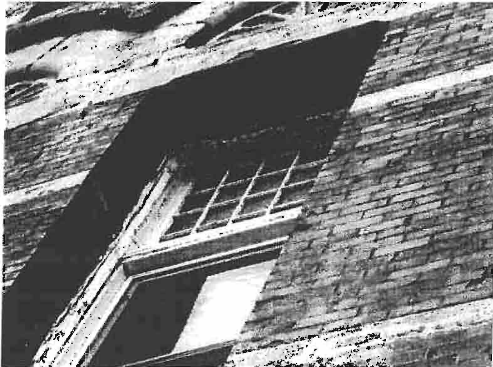
Photo No. 10: Wall Moved Outward. Caulking Joint Broken. (2014-05-23)
